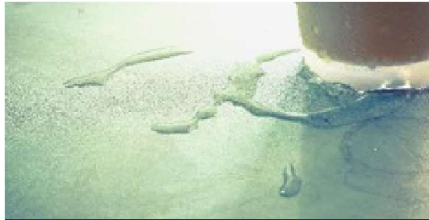
SURFACTANT LEACHING/WATER MARKS
