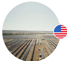
Solvay Solar Facilities United States
